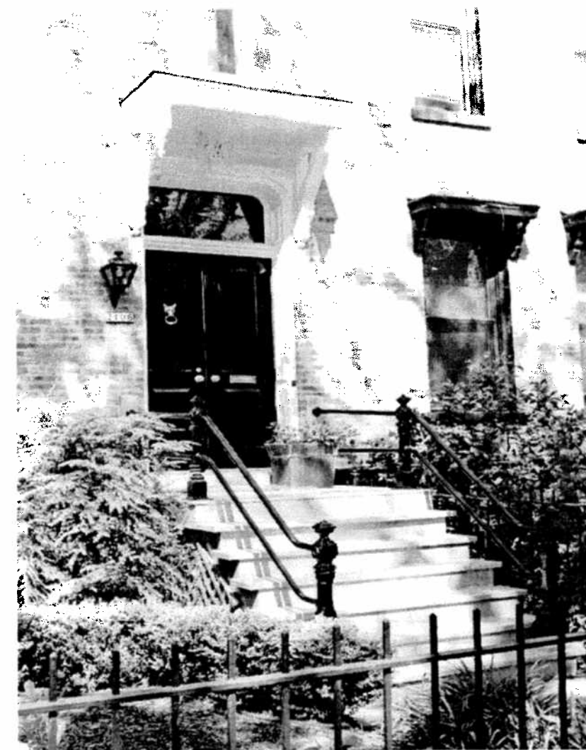
Above: The entrance to 2106 N. Fremont has a wooden pent roof with carved wood brackets. Left: 2106 has a front stoop with wooden steps and cast-iron railings leading to a wooden double door set within a round-arched frame with transom.
